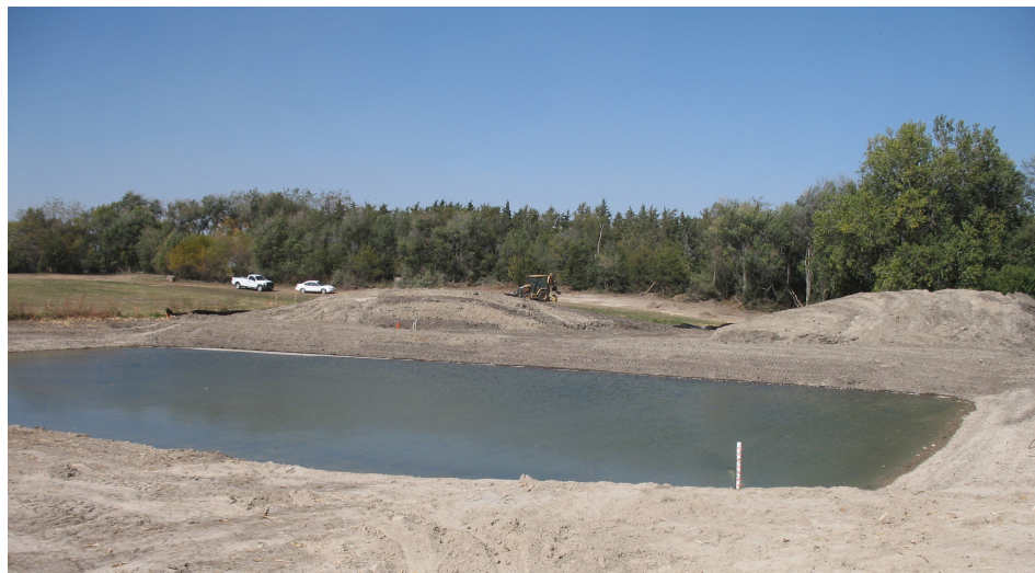
Pilot project — This recharge pit is part of a project to study return flows to the Platte River.
